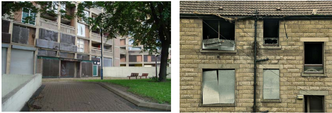
Figure 3, 4: Declined social housing estate with closed shops and empty/damaged housing units
